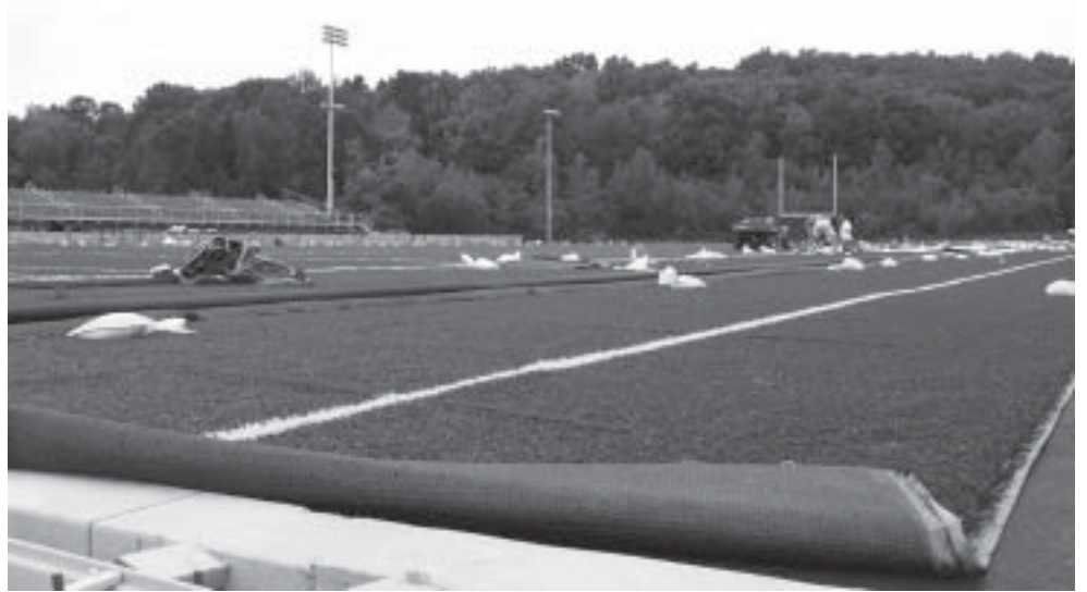
The construction crew lays and assembles the field turf in July for the multi-sport stadium in preparation of its fall semester opening.
